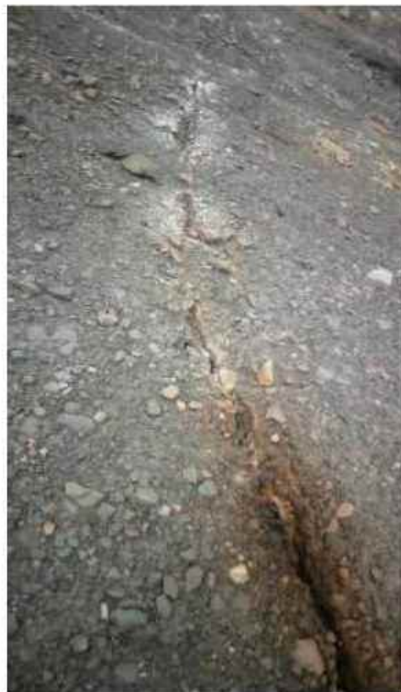
Figure 20: Fume cracks in the Bhulanbarari area.
